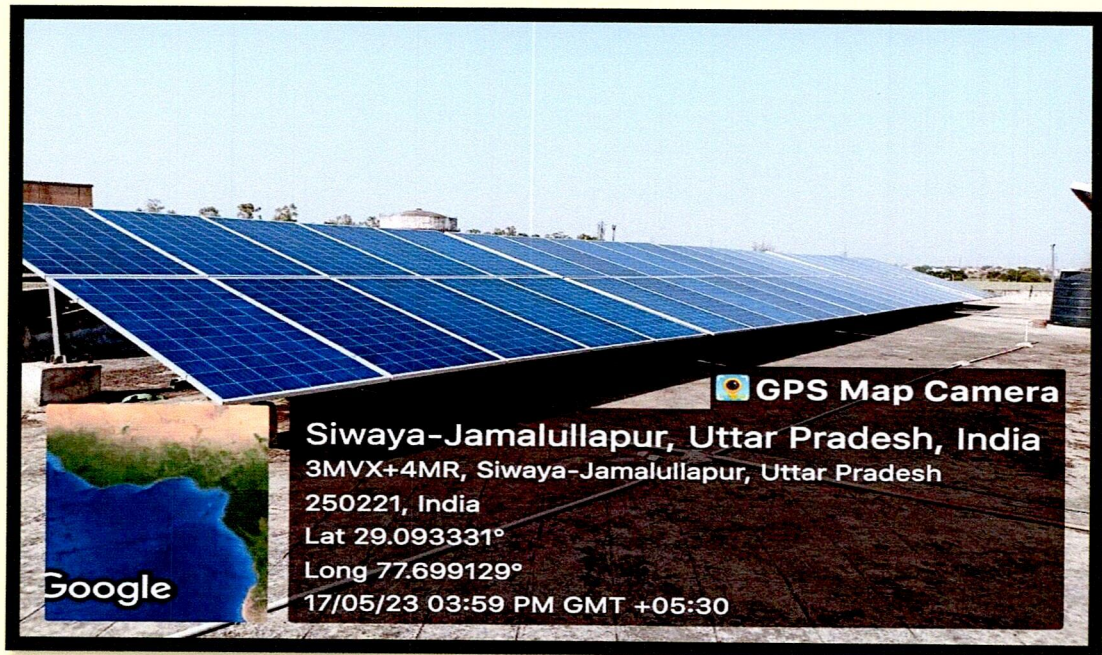
Solar System Panels installed on the roof top of University Buildings
